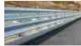
ROAD SAFETY GUARDRAIL
